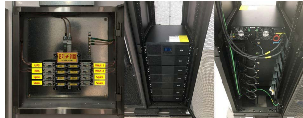
Fig. 8. Main power and UPS rack.
